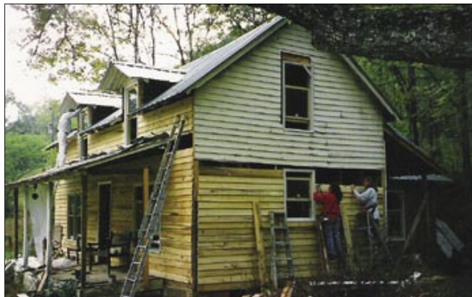
While renovating the house, from left, Carl Rasmussen and Linnie Boaté — David's uncle and mother — help Sharon remove old plank siding which was later reused as subflooring.
