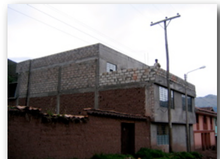
The nearly completed Josephine House. My room is directly below the man holding a bucket.
