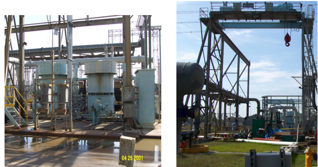
Fig. 10 1100 horsepower vertical circulating water pump / motor installation.
